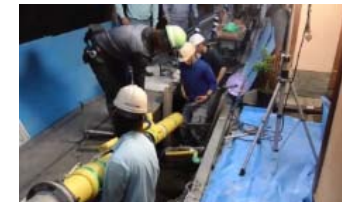
Solving ageing pipe issues
