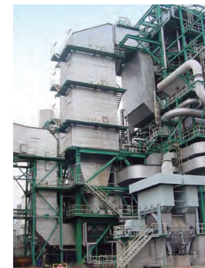
Flue gas denitrizer
