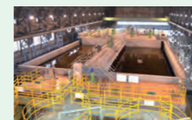
Motoyama AMD treatment facility at Toyoha Mine
