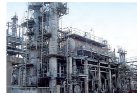
Flue gas desulfurizer
