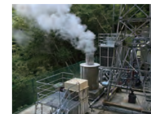
Shimoda Onsen Binary Power Plant
