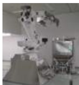
Intake automation equipment
